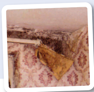
Damage to decorations caused by condensation
